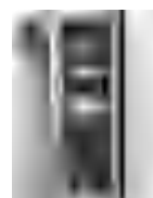
Auxiliary Power / AC-DC Distribution (including ATS)
